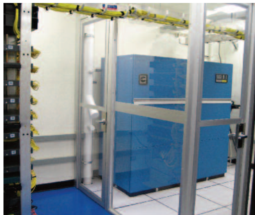
Make sure AC and CRAC units in the data center are positioned the move through the racks as efficiently as possible.
