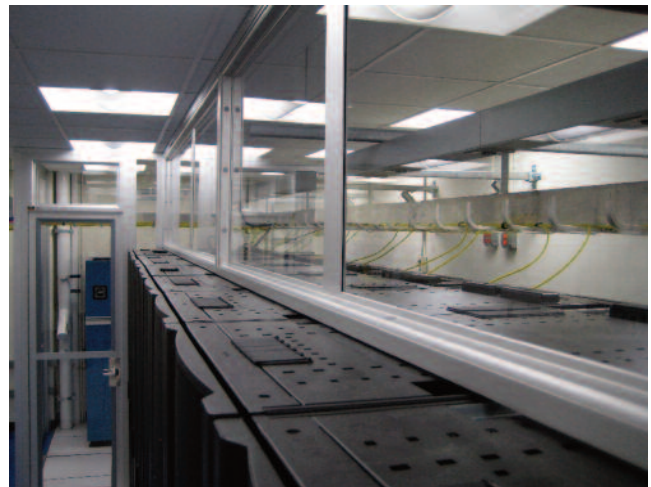
Good containment design means that hot air and cold are prevented from mixing in all locations, especially over the tops of the racks.
