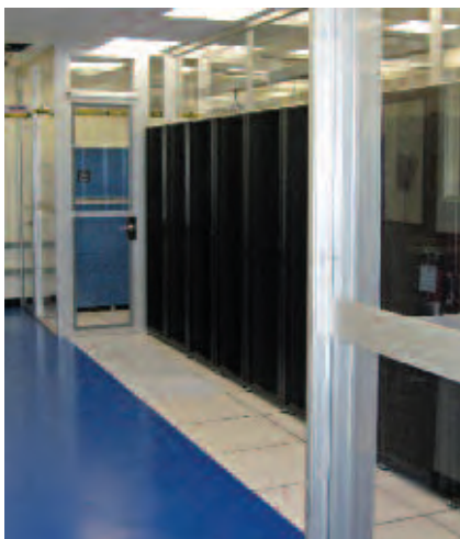
Data Center Partitions
