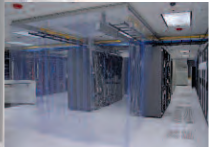
Strip Doors – End-of-aisle access is easy with strip doors. Strips come back together easily to limit air loss from one area to another.
